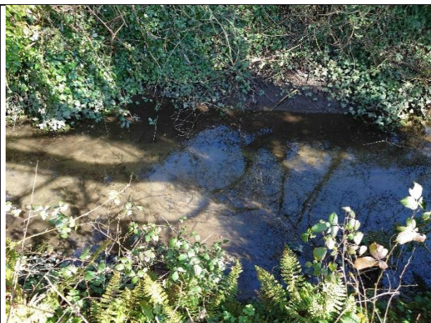
T22 – heavily silted side drain adjoining Thurstianstown Stream
