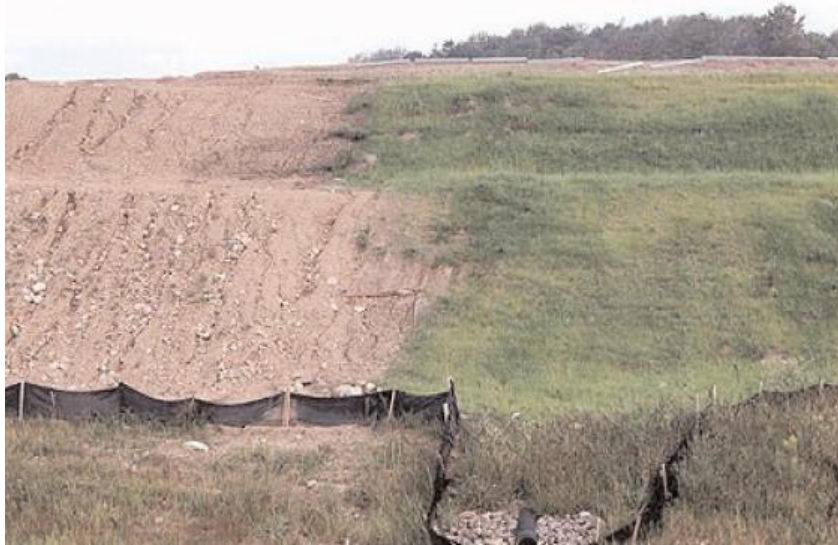
Figure 5.1: Before and after seeding. Erosion gullies visible on non-vegetated slope (Source: CIRIA C648)
